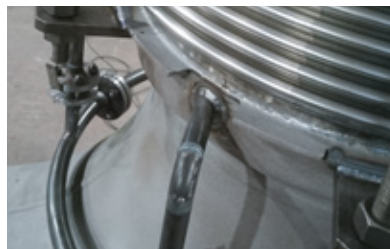
Ring line for the injection. This prevents the bellows becoming carbonised and reduces the bellows temperature
